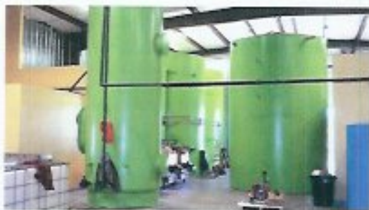
Used cooking oil is one of the feedstocks processed into biodiesel at Rocky Mountain Biodiesel Industries. The 3 MMgy biodiesel plant is located in Berthoud, Colo.
